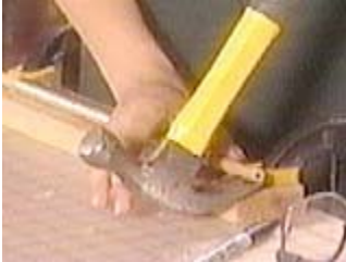
After drilling, use a hammer to pry the tube and doweling up
